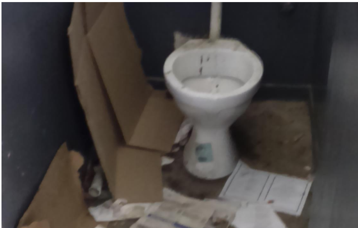
Toilet in Poor Condition: High numbers of learners per maintenance staff member is one of the reasons that nearly half of learner toilet blocks are in poor conditions.
