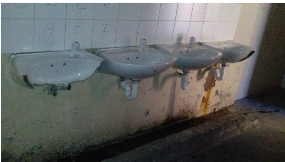
Broken Taps: While taps are generally present they are often broken.
