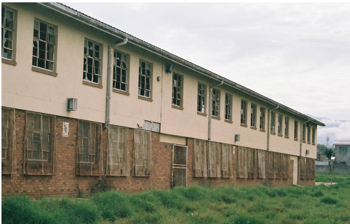
A Wing of Broken Windows: The entire top floor of this Cape Winelands secondary school has broken windows. Auditors were told that no classes are taught in this wing - local gangs come freely onto the premises and throw stones into those classrooms
