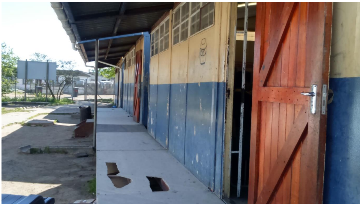
Disrepair: Many schools surveyed in the audit have not received significant infrastructure upgrades since before 1994.
