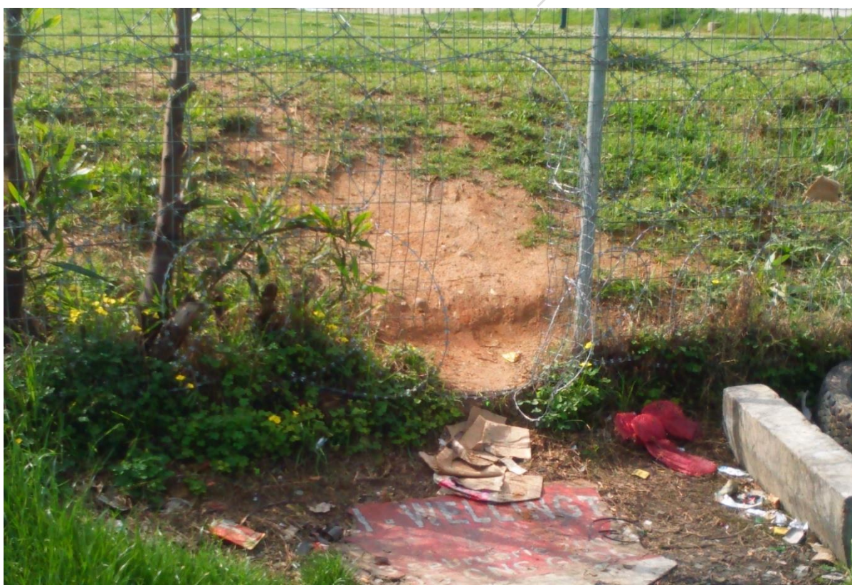
Holes in Fencing: This relatively newly-built secondary school already has holes in its wire fence; staff can't control who comes in and out, and the school lacks funds to keep repairing it. The school has no security guard.
