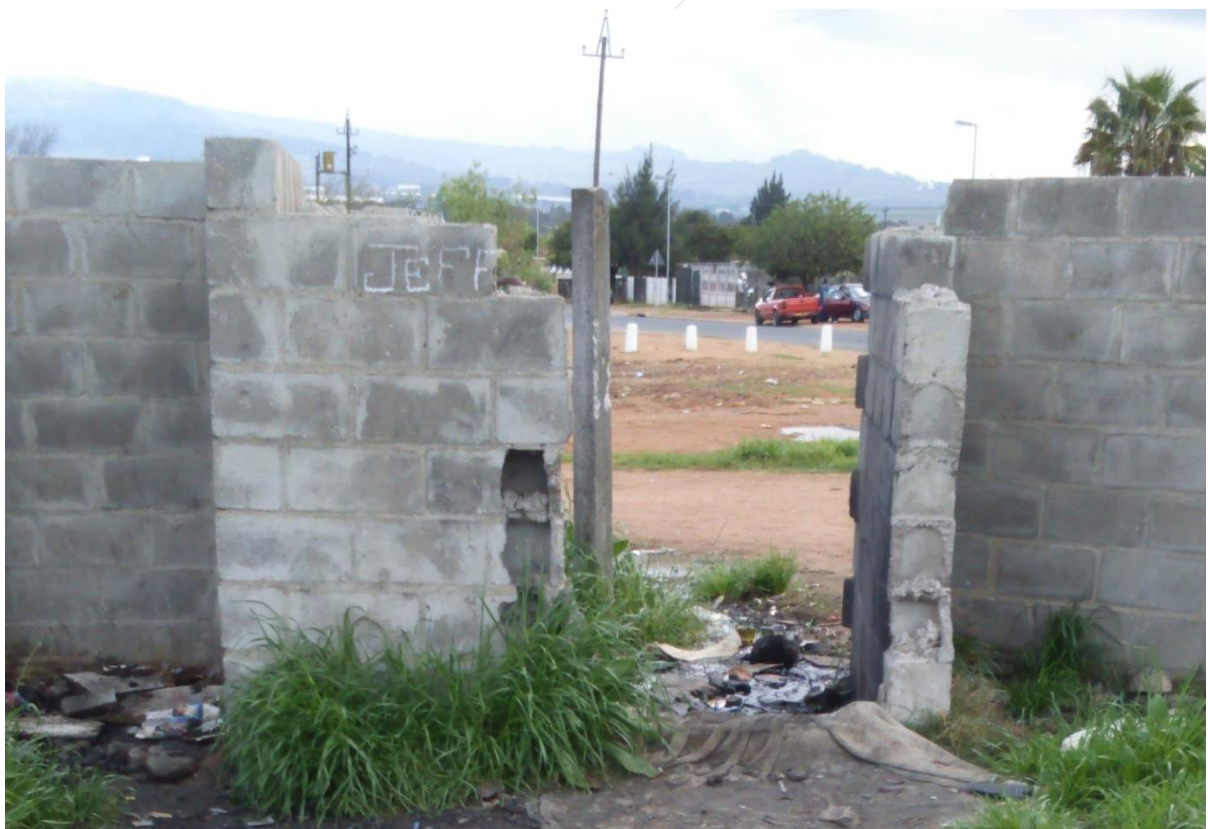
A Broken Fence is No Fence at All: This secondary school effectively has no fence at all – the perimeter is completely open, and auditors were told that local gangs often come into the school.
