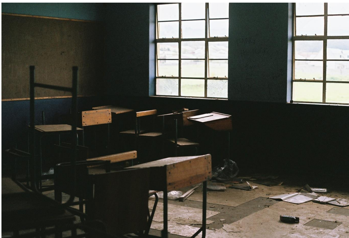
Abandoned Classrooms: Constantly in disrepair due to vandalism, the leadership at this Cape Winelands secondary school has abandoned this classroom.
