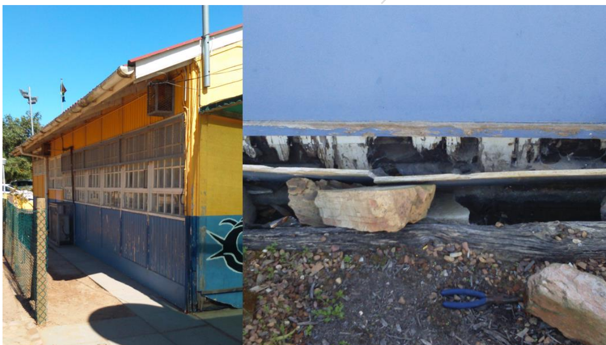
Partially Inappropriate: This rural school is partially built of wood. Many schools in the Western Cape are partially or wholly these types of “plankie” structures. Many are excluded from the Norms and Standards regulation because not all of the structures at the school are of this type.
