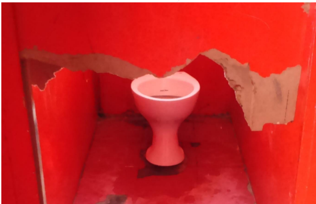
Broken Doors: The audit found that more than a third of toilets surveyed lacked doors that can be locked – the violates learners’ rights to dignity, privacy and safety.
