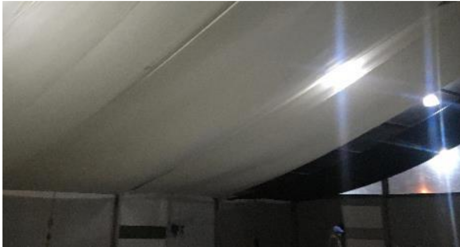
Figure 69: Poor ventilation resulting in condensation and drooping ceilings at The Haven Tent 2, 26 April 2020 (Source: Reverend Annie Kirke)
