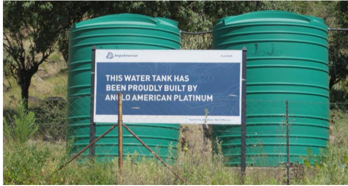
Above: Two of the lower Anglo JoJo tanks.
