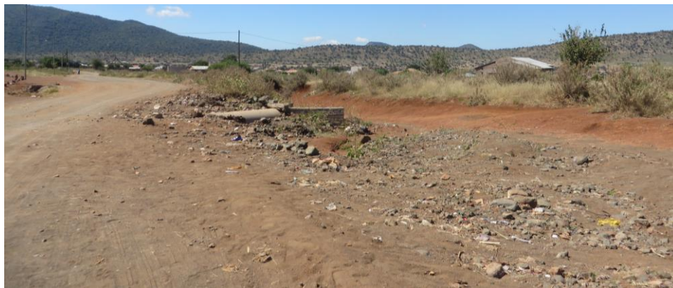
Above: The road in poor condition at a culvert.
